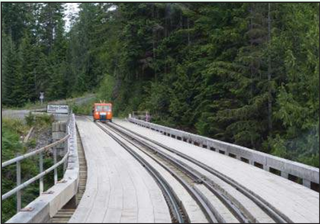
Above: The Storey Creek Bridge crosses over Canadian Highway 1 which is used by both the log trains and logging trucks.
