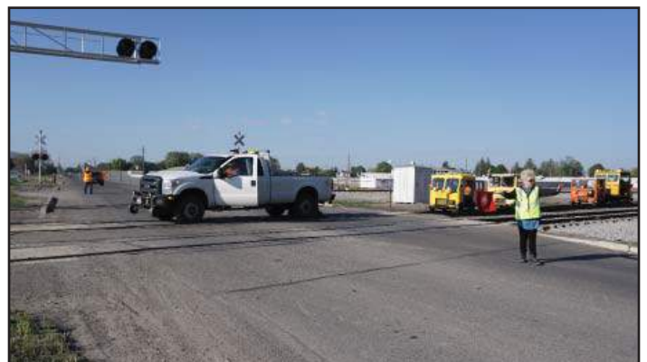
Right: Sean Crowe maneuvers his hi-rail truck on to the Hiland Avenue grade crossing as Dee Berg and Sue Pardee provide flag protection.
