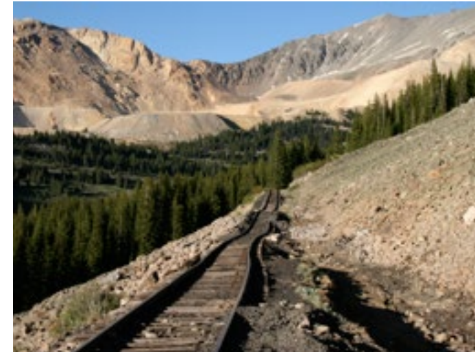
Extremely twisted track halts the excursion at the Devil's Tangent talus slope.
