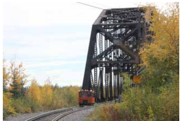
Located at Milepost 413 the excursion crosses over the Tanana River on the Mears Memorial Bridge. The 700 foot long structure is one of the world's largest single span truss bridges. It was built in 1923.
