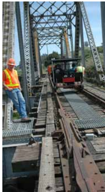
Danny Mihelcic supervises the motorcars crossing the Petaluma River on the 180 foot long Haystack swing bridge. The bridge was built in 1909.
