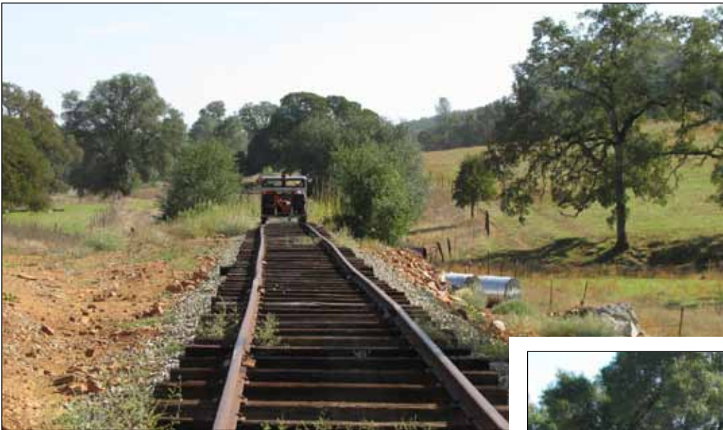
After lunch and heading for Shingle Springs the motorcars pass over the Latrobe Creek washout site. The roadbed and rails were replaced last May. Track reconstruction was performed by Placerville and Sacramento Valley Railroad volunteers.
